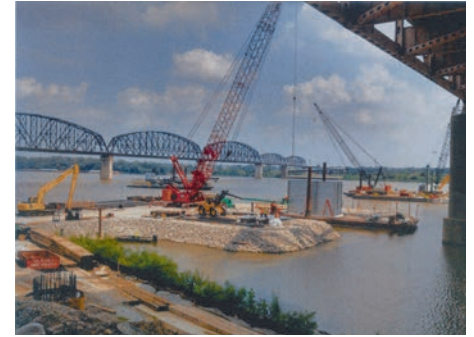
Walsh Construction installing the bin-wall at the Downtown Bridge Crossing in Louisville, KY
