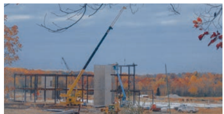
G & M Steel Erectors setting steel at the Perry County Hospital project in Tell City, Indiana
