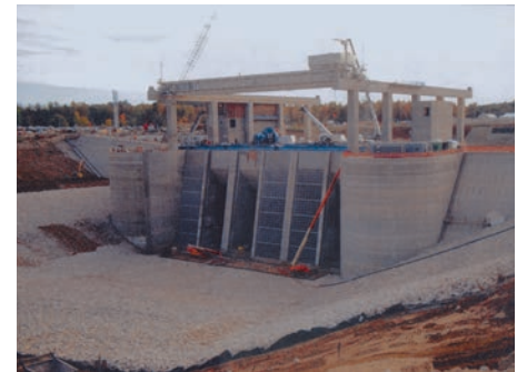
Inlet side of the Cannelton Dam Hydroelectric project in Hawesville, KY
