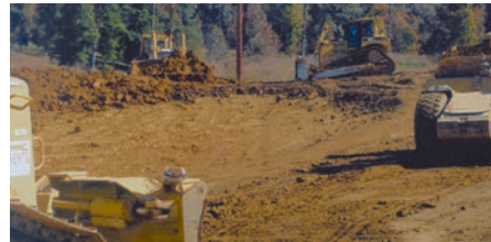
Parkway Construction working on the approach ramps at the Dawson Springs, KY exit on I-69
